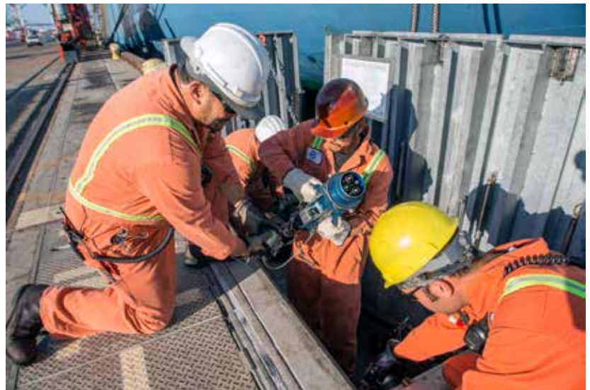
Ports are helping to reduce emissions from ships, including cold-ironing systems such as the AMP shore power program at the Port of Los Angeles. Photo courtesy of the Port of Los Angeles.
